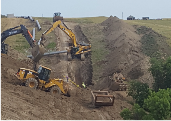
Storm Drain Infrastructure, Cherry Creek Community
